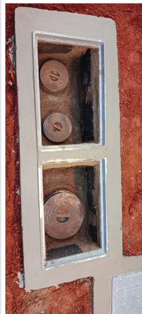
Step 7: Make provision for 2 inspection points/manhole covers - 600mm by 450mm as shown in the picture
